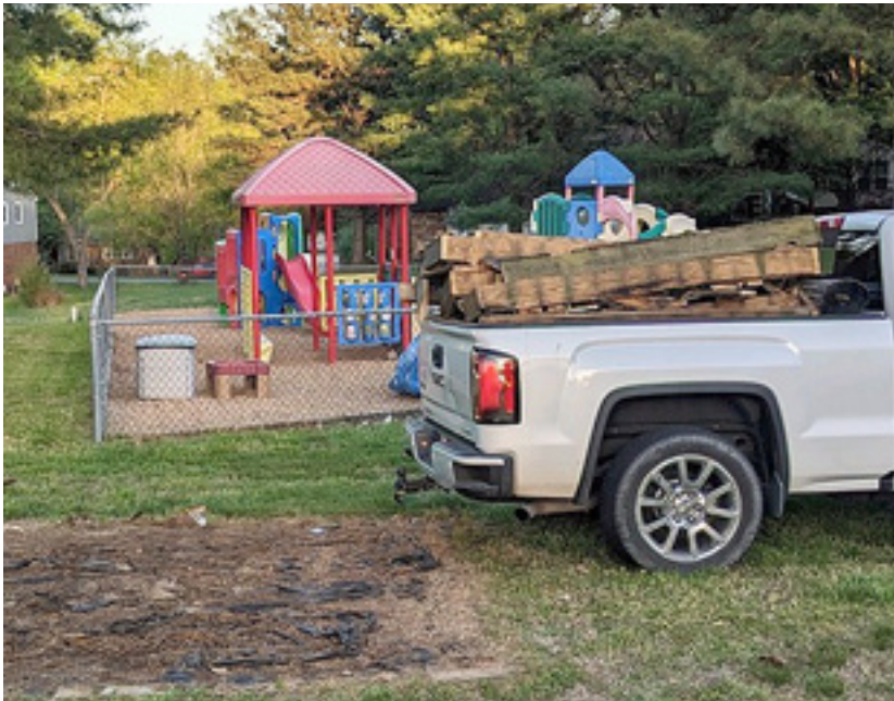
The demolished stage loaded onto C.W.’s truck and bound for the county dump.
